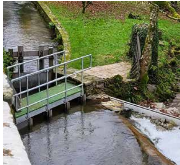
Bridgetown Smolt Grill & Smolt Pass (to prevent Salmon Smolts entering the leat)
